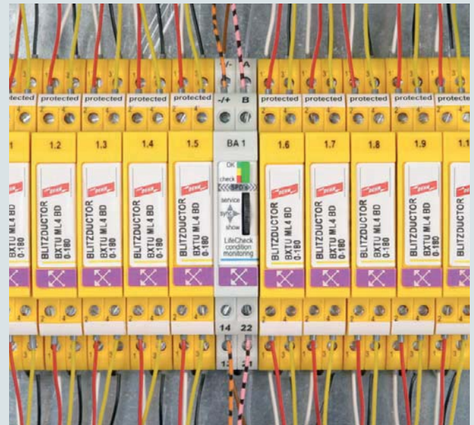
DEHNrecord Condition Monitoring-Einheit in der Installation.
